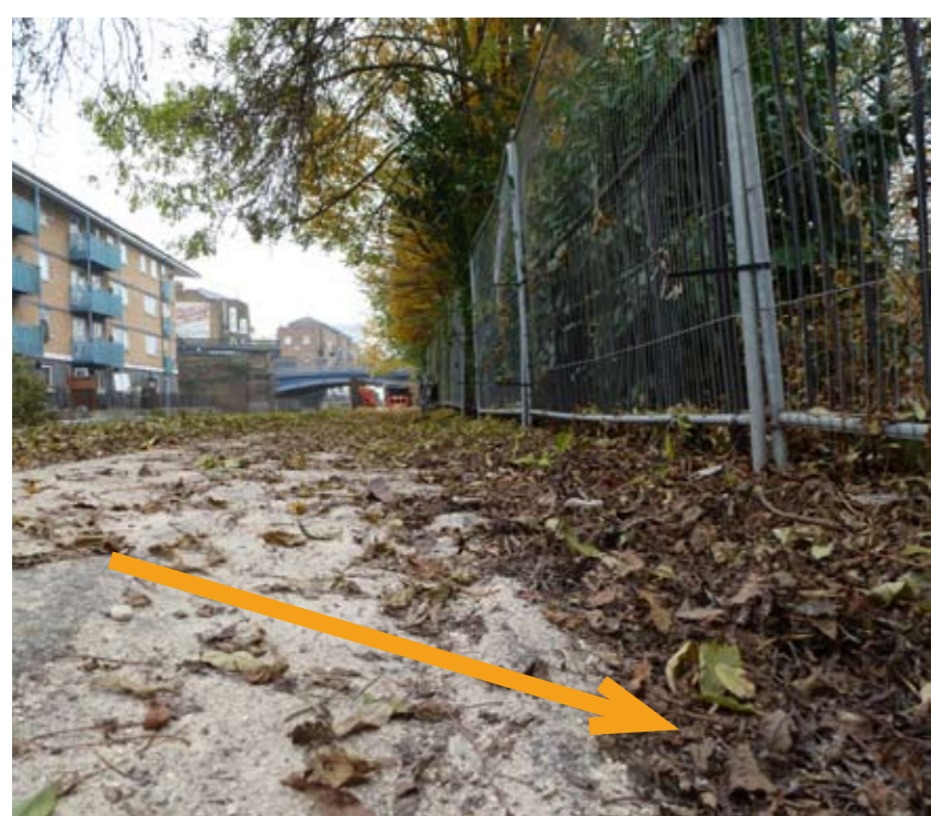
5 Uneven surfacing that sometimes slopes towards the canal or offside.
